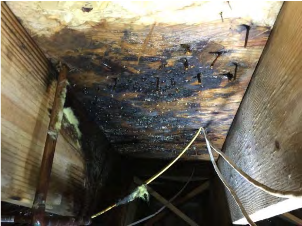
Because of moisture, MOLD can easily grow and spread in crawl spaces.
