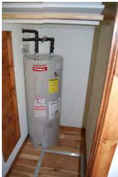
Typical Water Heater
